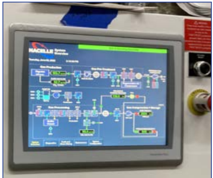
RNG process monitoring
