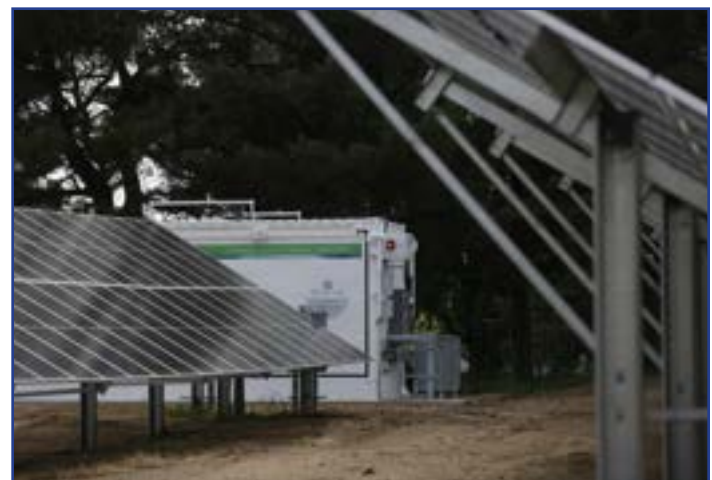
Battery storage with solar arrays
