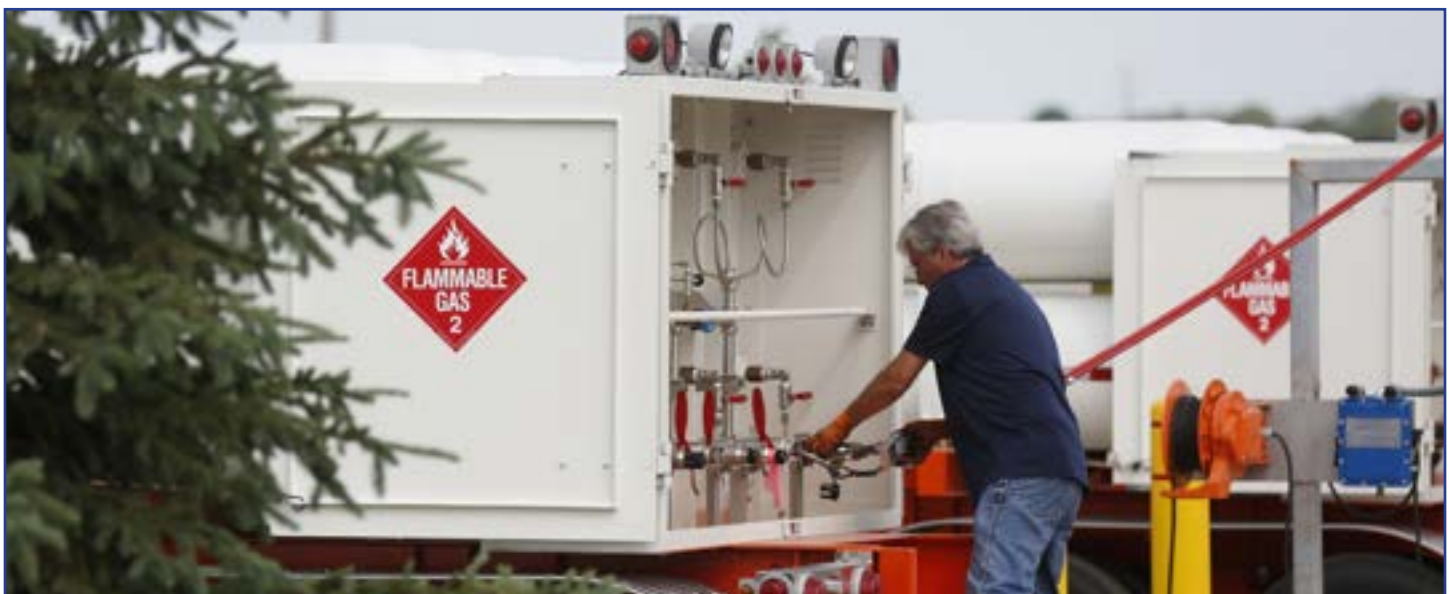
RNG transfer to truck for transport to pipeline injection point, EnTech Solutions, Town of Springfield, WI
