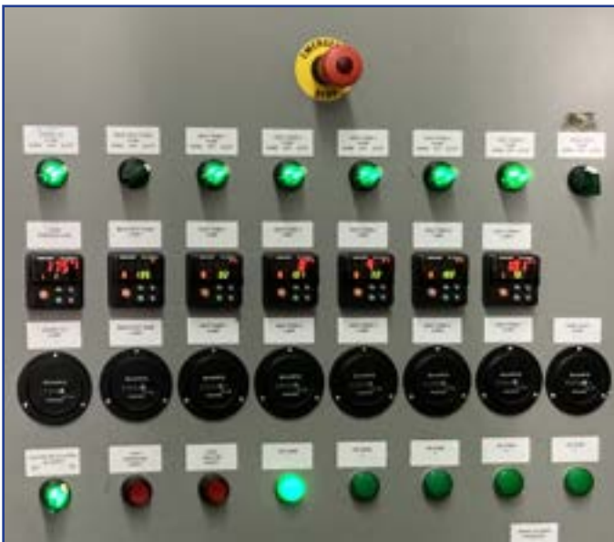
Digester heat pump monitoring
