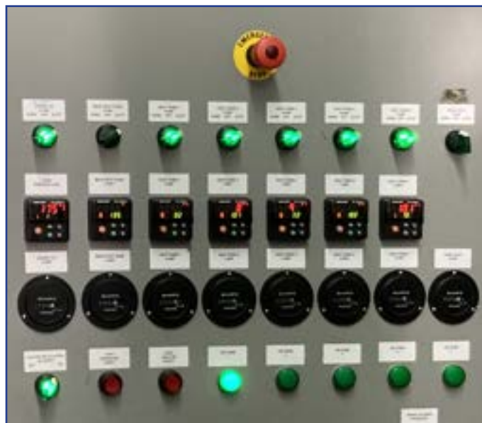
Digester heat pump monitoring
