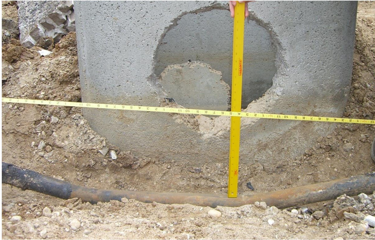
Displaced steel main (not located)
