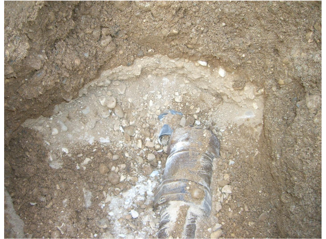
Compression coupling about 12' away from catch basin
