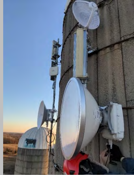
Above: Wireless Access Point being installed in Green County with CARES funding
