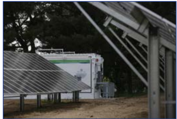
Battery storage with solar arrays
