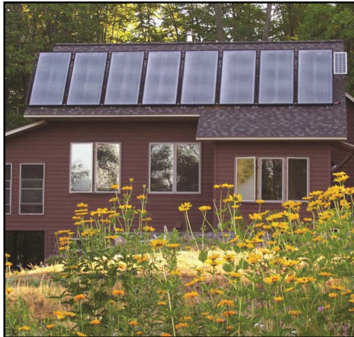
Residential solar hot water collectors
