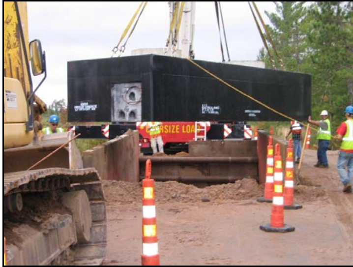
138 kV XLPE project – Pre-fabricated top half of vault being lowered into trench.
