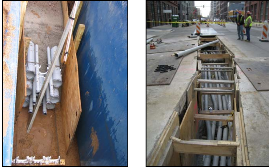
Figure 11 Examples of XLPE Conduit Assembly
