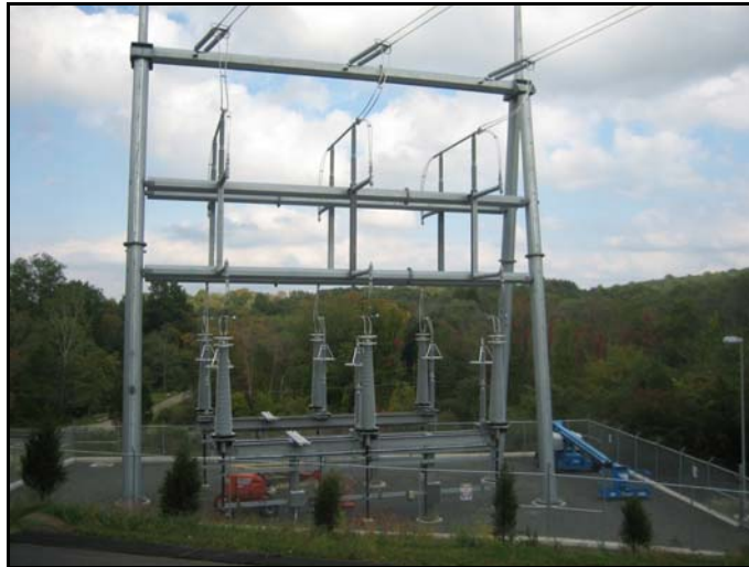
Figure 7 Small Transition Station
